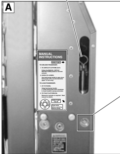
Manual Backup Pump
